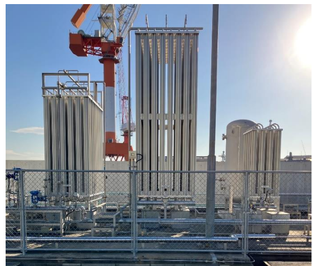
Figure 4. Air-heated vaporizers (HX1, HX2, HX3)
