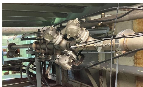
Figure 12. Gas detectors on outer pipe
