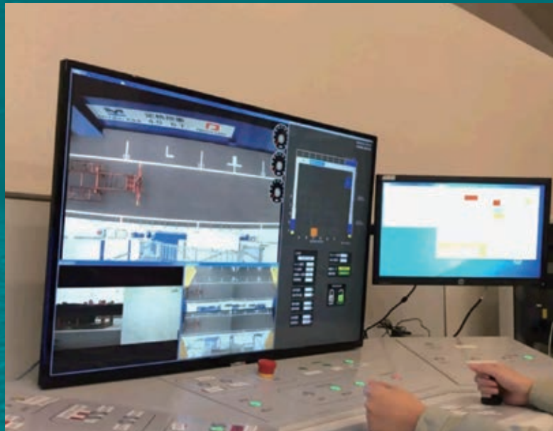
Remote Operating Console
